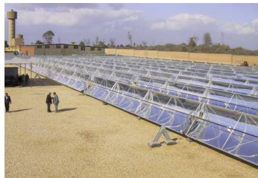
Fig. 12: Solar thermal process plant - steam production in chemical industry (source: Fichtner Solar GmbH, Germany)
